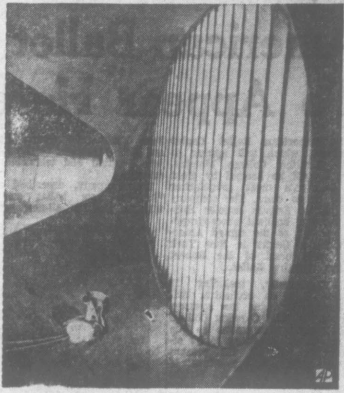
BIG BLOWER — Giant cone which can funnel a 3,000-mile-an-hour gale points to steel vanes in Air Force supersonic wind tunnel being built at Tullahoma, Tenn.
