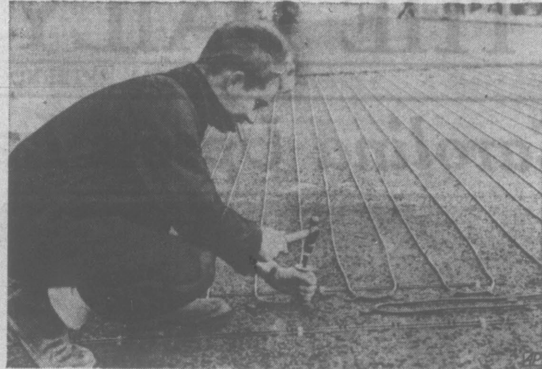
HEAT FOR HIGHWAY — An electrician fastens down part of a special heating cable to the road surface of highway near Kingston, Eng. The final layer of asphalt is laid over the cable which helps to prevent freezing on the road in icy weather.
