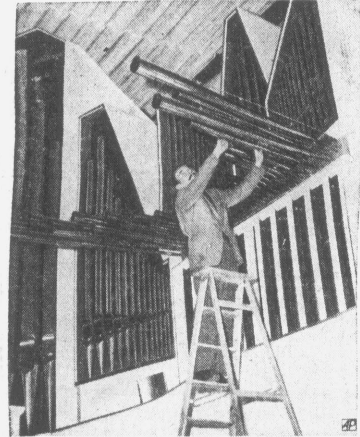
MUSIC FROM THE SIDE—A worker fixes organ pipes to the new organ under construction at Trinity Church in Hamburg, West Germany. Some of the pipes are placed horizontally to produce a trumpet effect.
