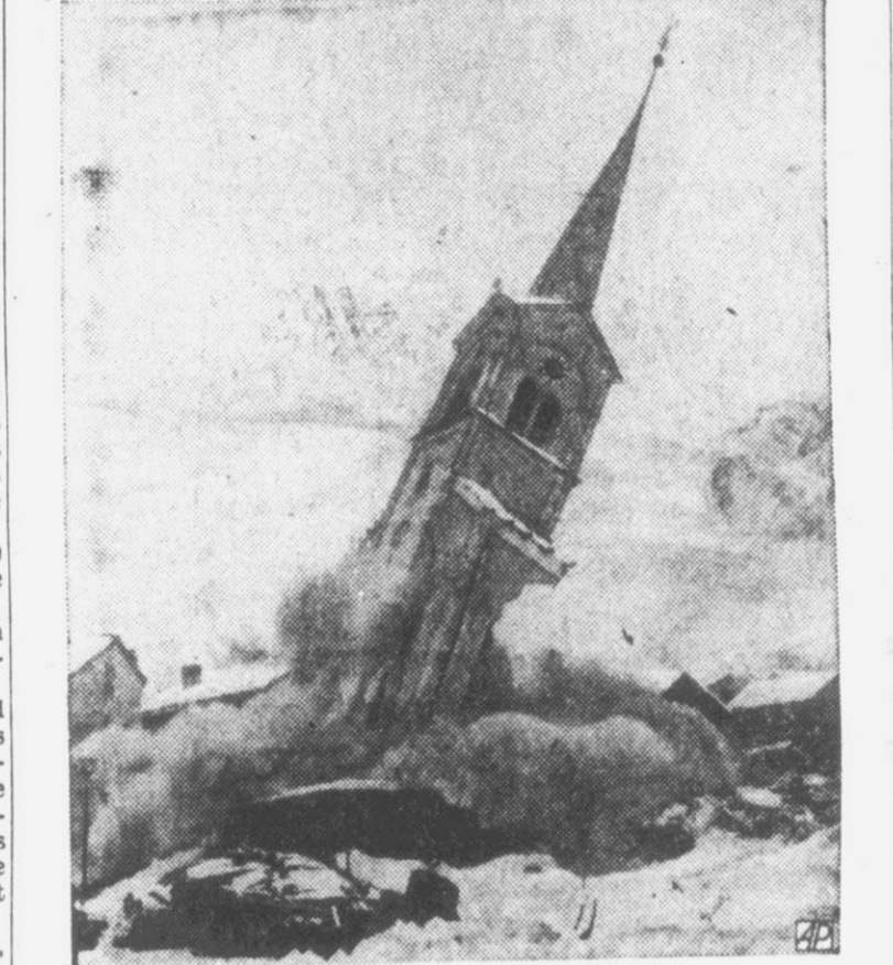
EARTH BOUND — Steeple of the parish church of Saas Fee in southern Switzerland crashes to ground after being blown up to make way for new church edifice.
