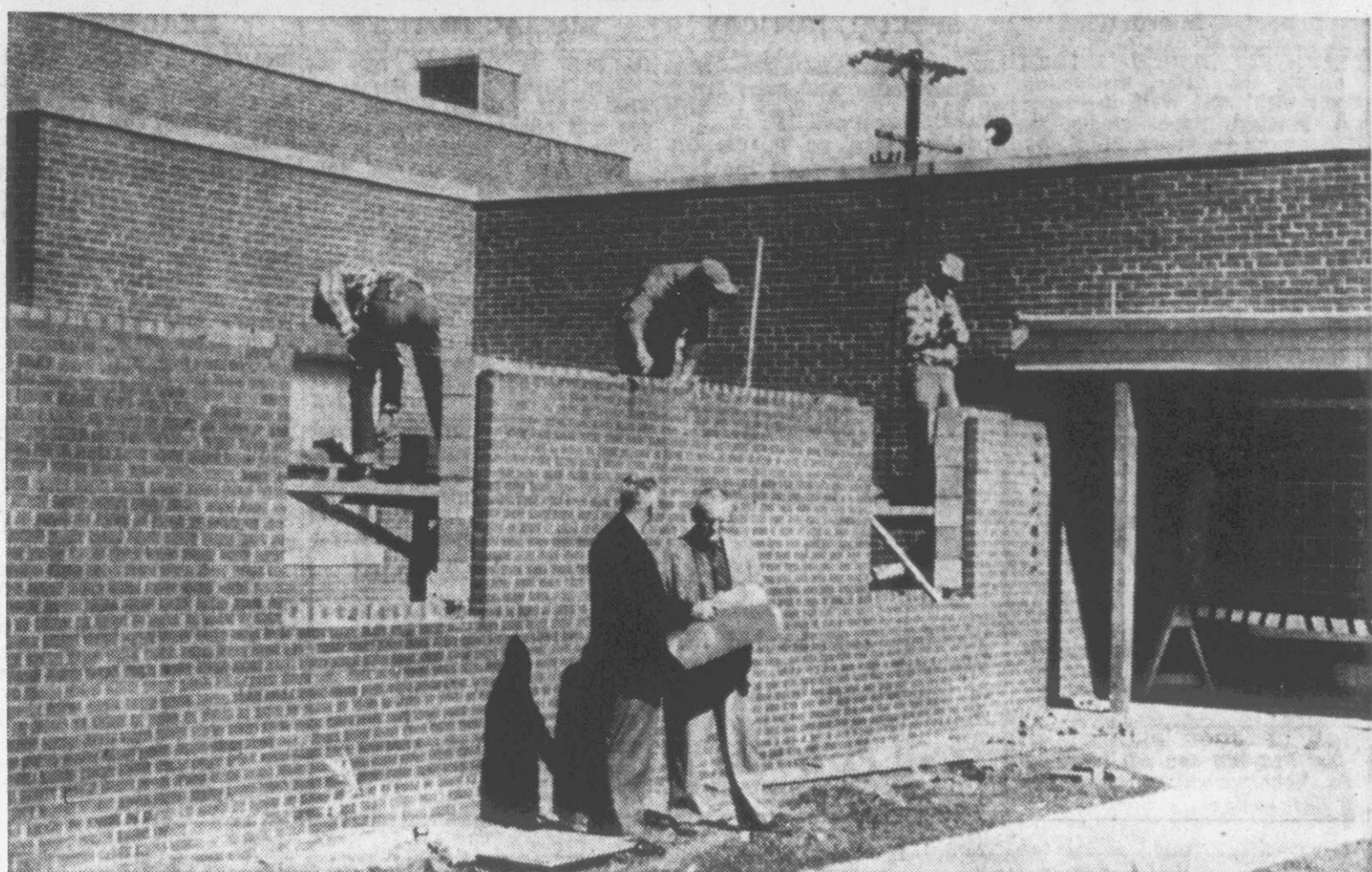
MOOSE LODGE ADDITION UNDER WAY. Sec. Baldree and Building Committee member Stauffer go over plans.
