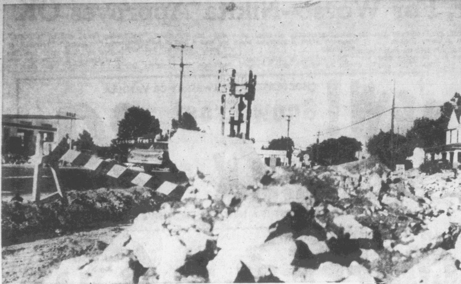
CURB AND GUTTER —The busy intersection of U. S. 264 and U. S. 17 is getting curb and gutter at Chocowinity. The installation will widen the intersection considerably and provide for better turning by vehicles. The Highway Commission also plans to install traffic control signals at Chocowinity. (Reflector Staff Photo)
