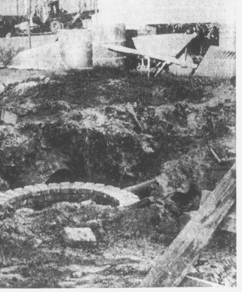
"DRAINAGE PROJECT" on Clark Street between 10th and 13th Sts. will be completed in about 15 to 20 working days, according to City Manager Leonard Bixham. Bixham said the much needed drainage work is being financed as part of the bond issue for drainage work. Work was started on the project last Monday. (Reflector Staff Photo)
