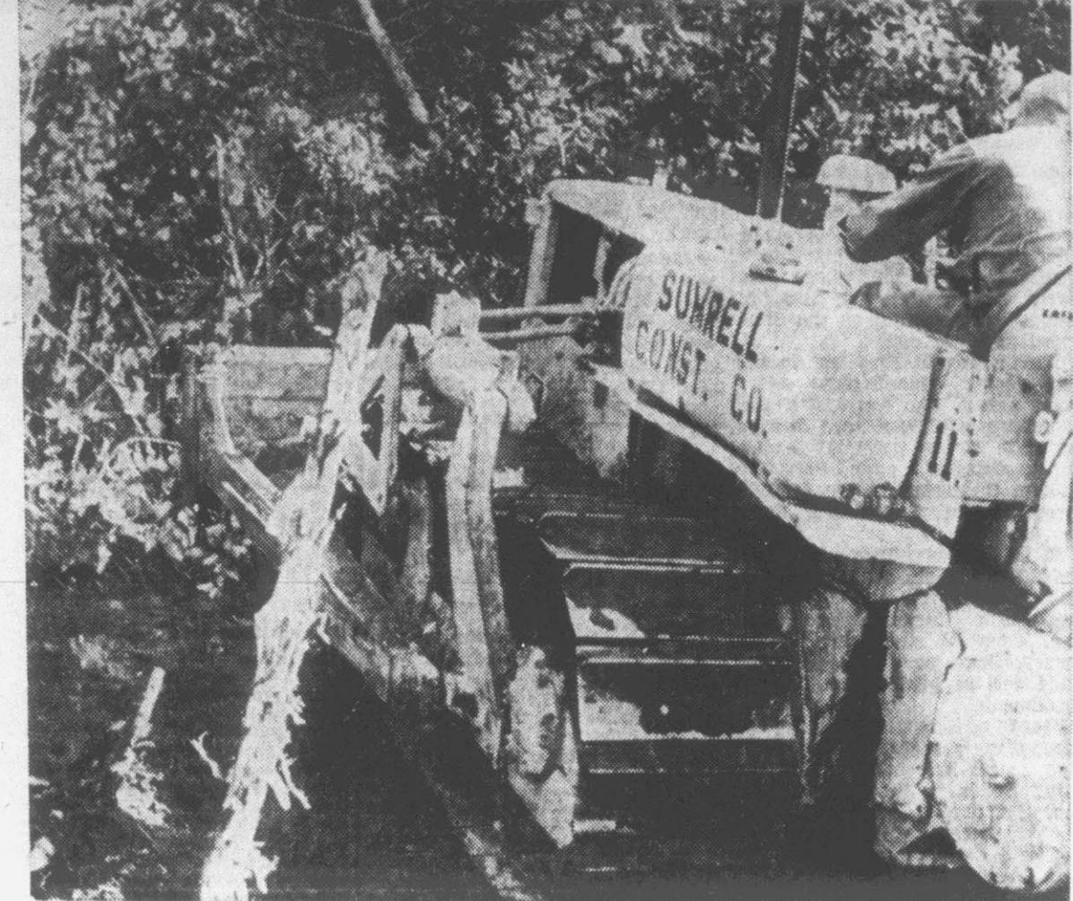
CLEARING LAND . . . for the Greenville Police Department's future Club House and pistol range improvement is a bulldozer from a local construction firm. According to Chief S. G. Gibbs the firm is donating the machines and operators to clear the land and dig drainage ditches on the property. The local department is sponsoring a dance and a variety show October 2 at ECC's Wright Building to raise money for the project. Chief Gibbs said the department was given all the brick and timber from the old Norfolk and Southern Railroad passenger station which was torn down recently on Dickinson Ave. for use at the Club House and range. (Reflector Staff Photo)
