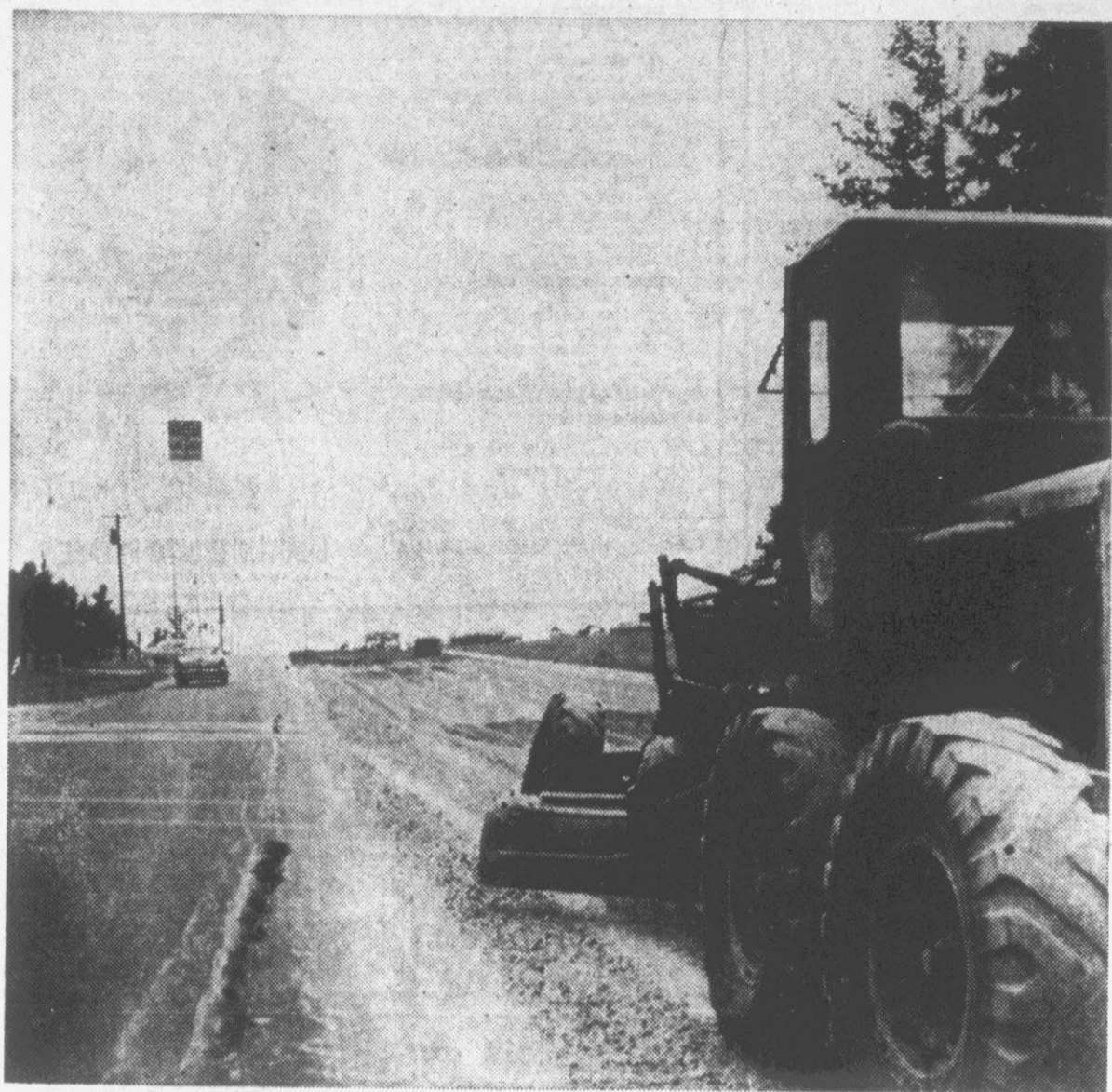
DRAINAGE PROJECT ... A road machine is shown at work on a drainage project on Elm St. across from Elm St. Park.
