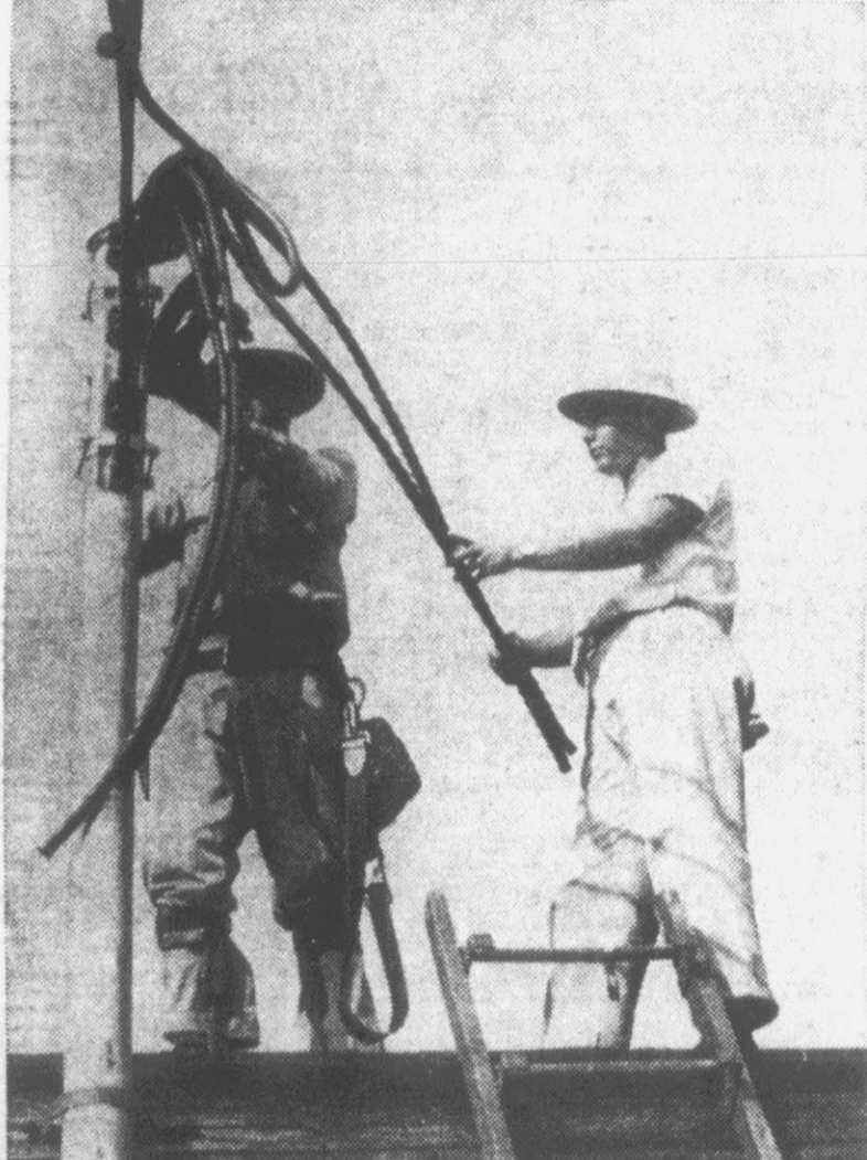
HIGH-VOLTAGE WIRING . . . goes into the temporary home of Farmville's newest industry, the Farmville Manufacturing Company.
