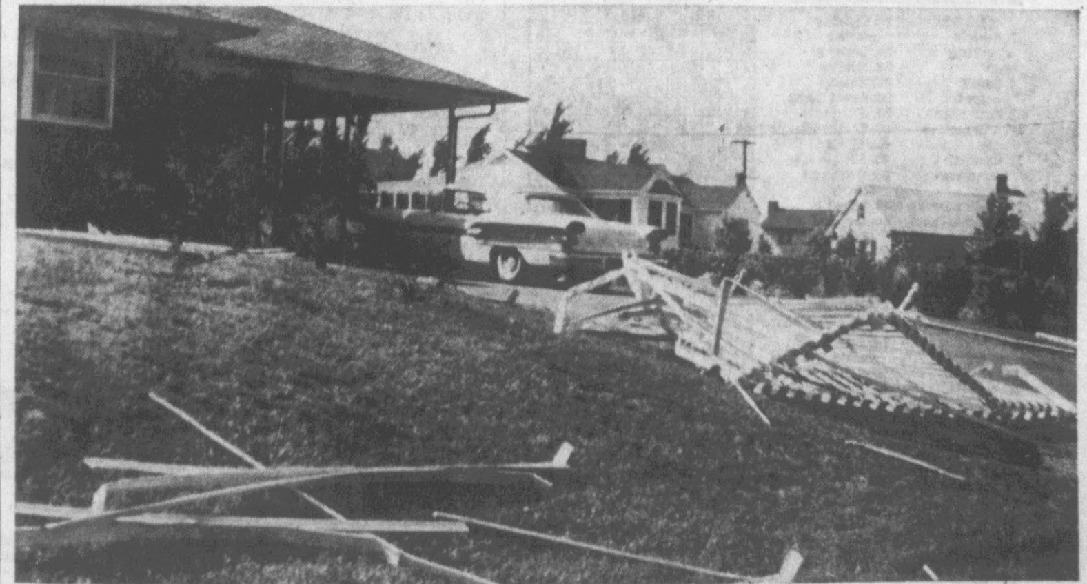
FREAK WIND . . . tore this aluminum awning from the rear of the house.
