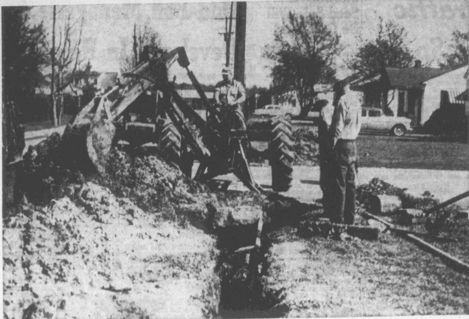
NATURAL GAS LINES BEING INSTALLED—Construction crews are at work in Farmville installing new lines for the North Carolina Natural Gas Corporation. The gas lines will bring natural gas into Farmville after being connected with a transcontinental pipe line. Streets on which the mains are being installed are Main, Lang and Walnut. (Reflector Staff Photo)
