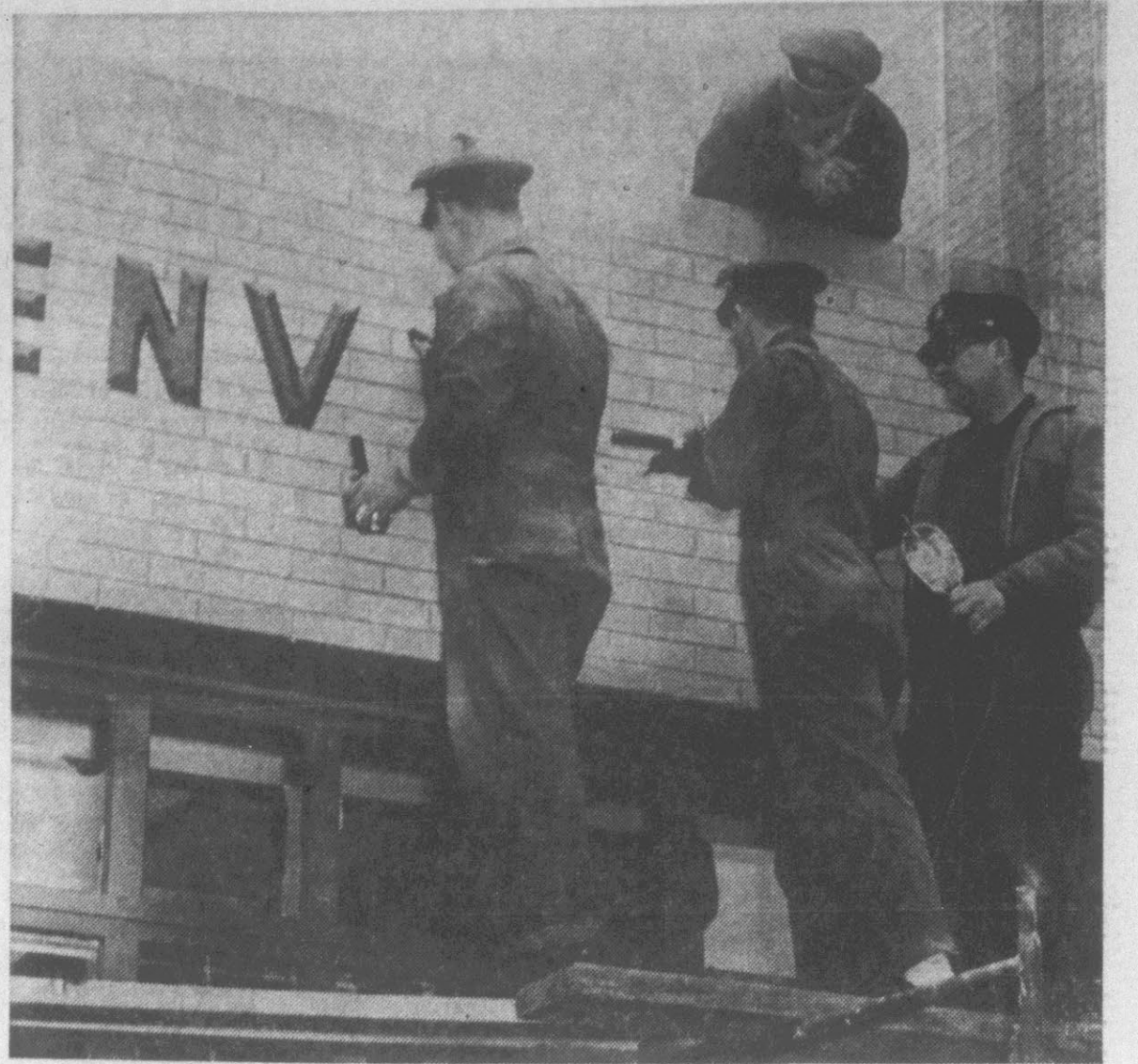
RESCUE BUILDING GETS SIGN—Firemen Ray Smith, J. Z. Garris, Alton Vincent and Claude Christopher (top) install a sign on the new Greenville Rescue Squad building. The annex to the fire station will house the squad's equipment. Dedication ceremonies for the new structure are expected to be held in the near future. (Reflector Photo by Rosalie Moore)
