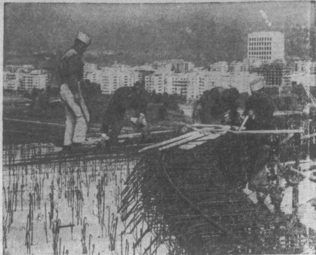
PREP FOR BIG GAMES — Laborers set up concrete reinforcements for arena under construction at Rome's exposition grounds for the 1960 Olympic Games. Arena will be air-conditioned and is to provide facilities for a record entry of athletes.
