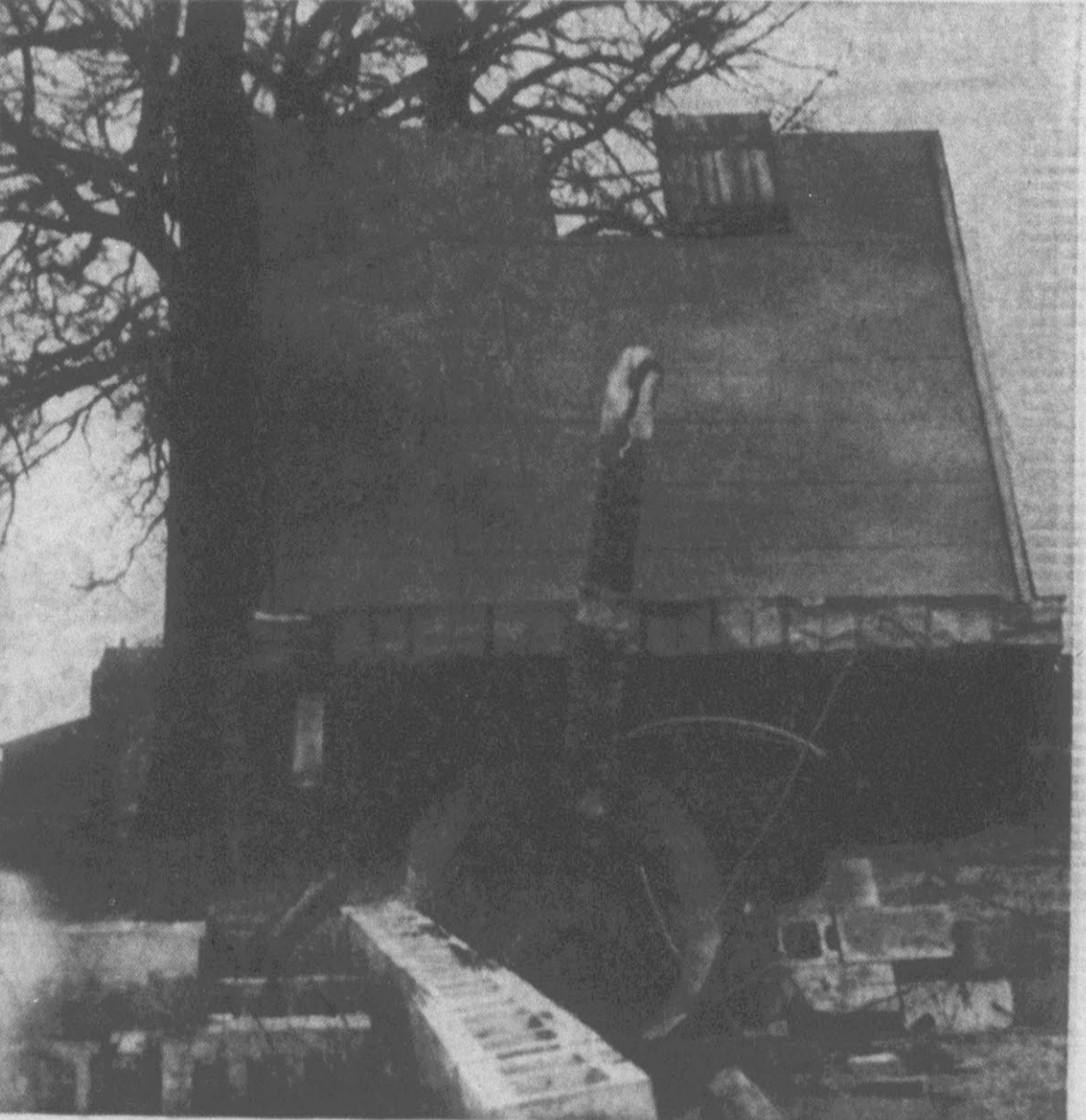
TOBACCO BARN IS OVERTURNED . . . as local wind storm hits on Falkland Highway.
