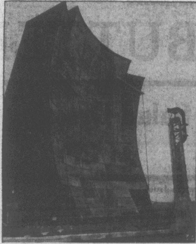
COLD PACK — Workmen caulk seams of face of 60-foot parabolic antenna, one of the "iron ears" of communications system that stretches 3,100 miles across Alaska.
