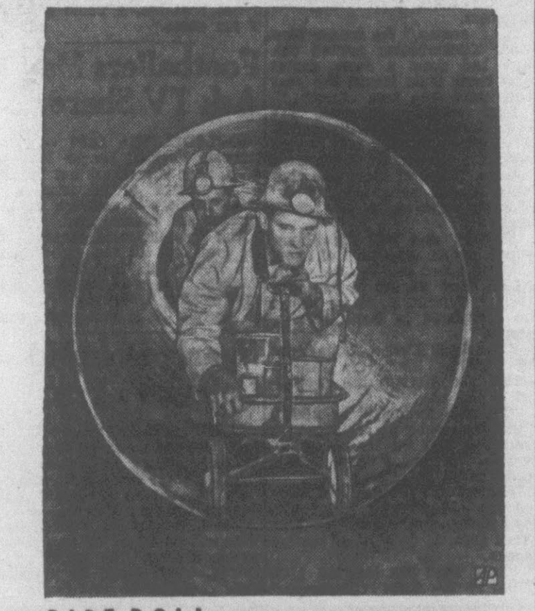
PIPE ROLL—Workmen use a toy wagon to transport their tools and materials through 48-inch diameter pipe tunnel being completed for Pittsburgh's sewage system.
