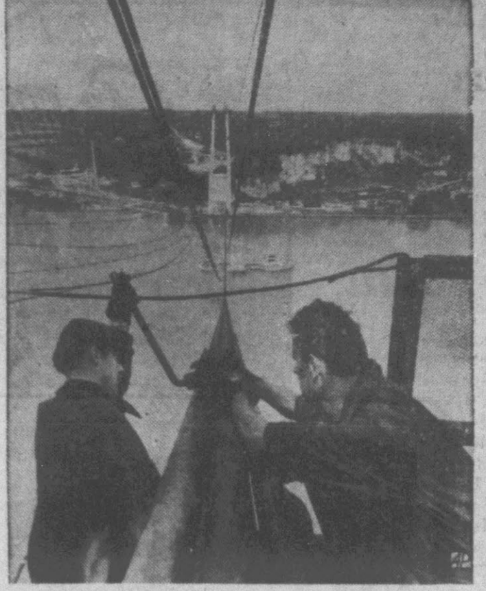
STEEL WORK — Workmen tighten cables for bridge under construction across Seine river at Pont Aude-mar, France. Bridge will be largest on European continent.
