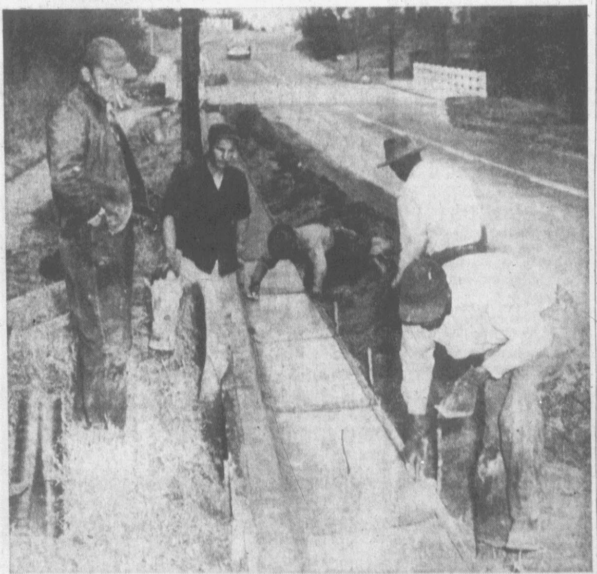
CURB AND GUTTER ON 14TH ST. — Workmen are installing curb and gutter on 14th St. from the railroad siding which leads into the college campus to Charles St. Completion of the 2,000 foot section will mean that the street will be curbed and guttered throughout the city. The work is being done under the city's contract and the city will be reimbursed by the State Highway Commission which maintains the street. (Reflector Staff Photo)
