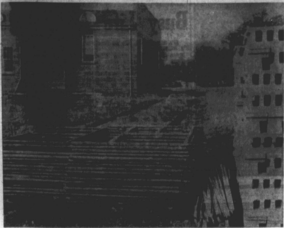
CONSTRUCTION ON CLASSROOM ADDITIONS AT THE WINTERVILLE HIGH SCHOOL . . . has already begun—to be completed in 28 weeks. (Reflector Photo)
