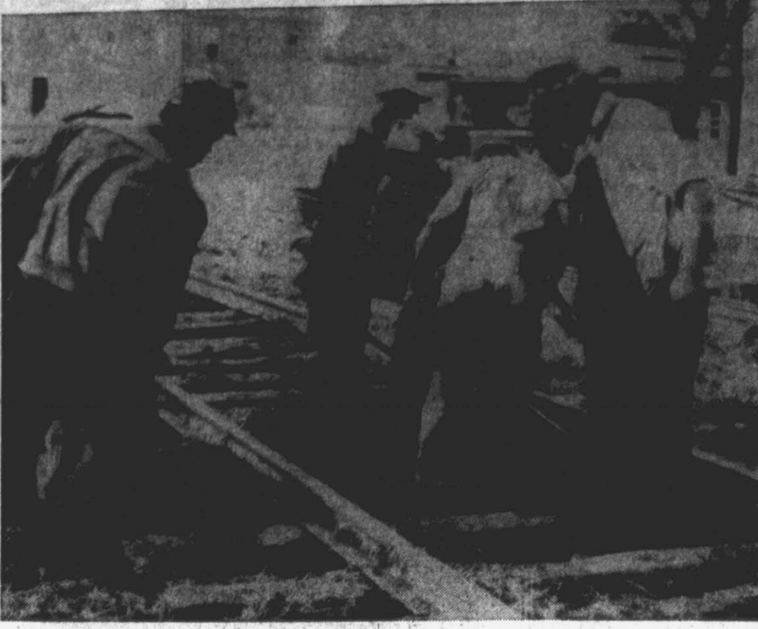
NORFOLK AND SOUTHERN CREWS AT WORK . . . spur lines removed by workers on Ninth St.
