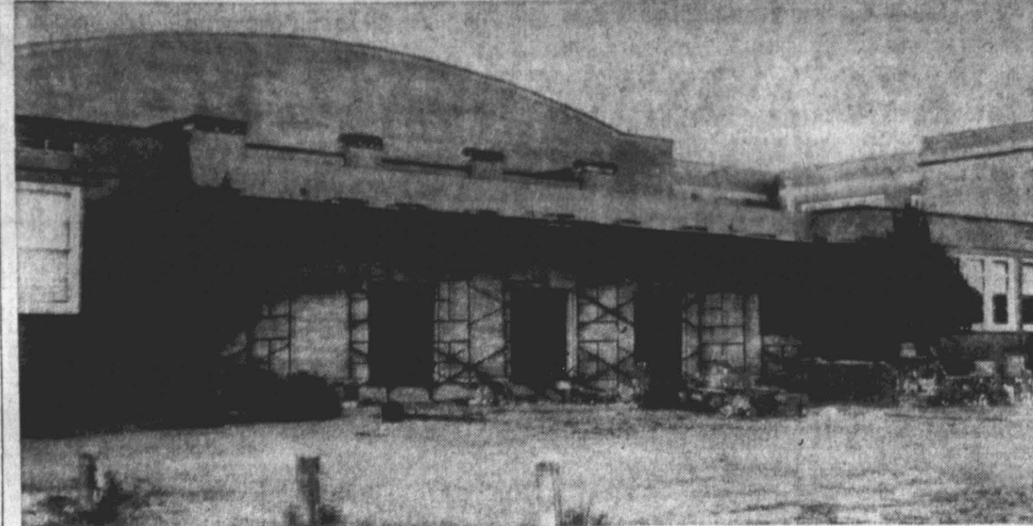
CONSTRUCTION CONTINUES —Construction of a lobby for Farmville High School's gymnasium is continuing and is expected to be completed by opening date of the 1958-1959 school year. What was formerly the gymnasium porch is being enclosed to provide offices for physical education personnel and to provide space for a concession stand. (Reflector Staff Photo)
