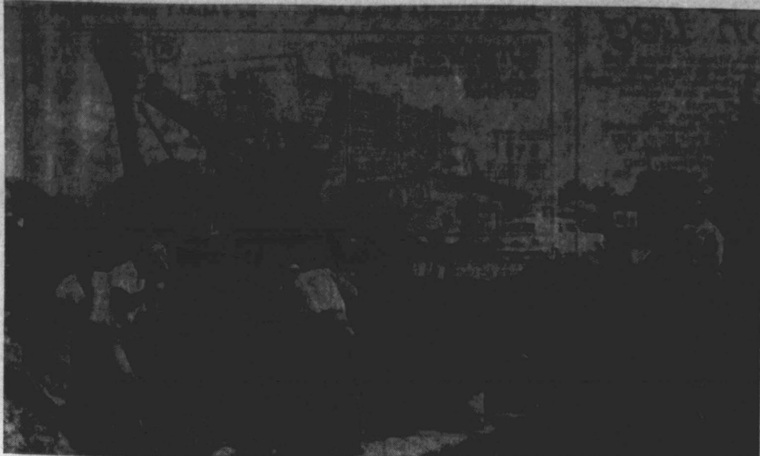
LARGE CRANE, WORKERS DIG DITCH FOR SEWER LINES . . . over five miles of pipe have been laid within Ayden city limits. (Reflector Photos)
