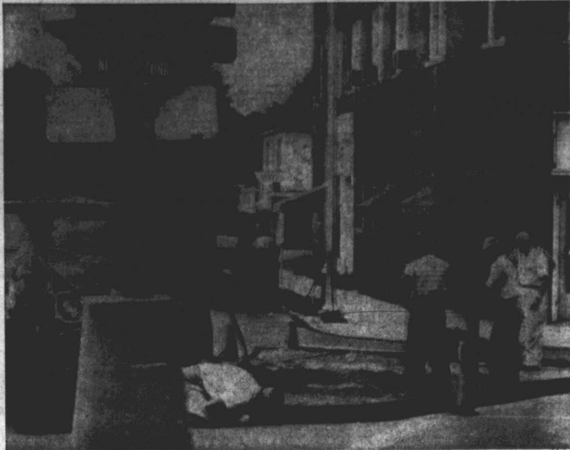
TRAFFIC ISLANDS—City crews are installing asphalt traffic islands at Five Points to aid in the channeling of vehicles at the complicated intersection. The areas which the islands will occupy were previously marked off with yellow paint. The raised asphalt islands will prevent autos running in the areas. They also provide safety islands for pedestrian traffic. (Reflector Staff Photo)
