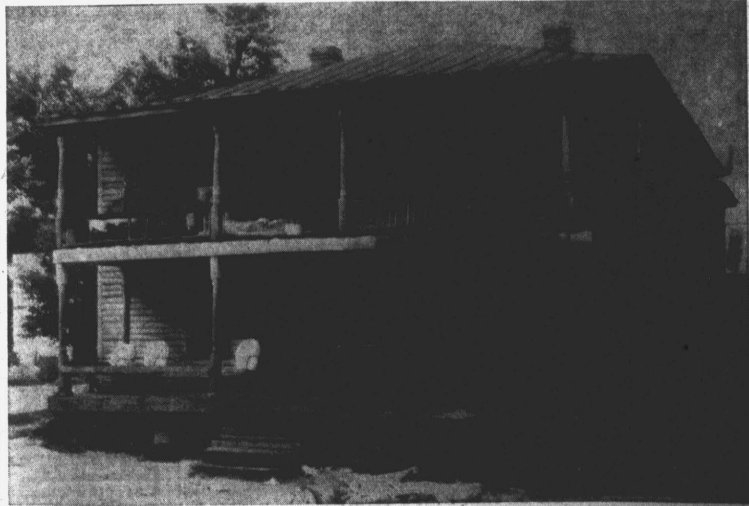
THREE ROOMS IN THIS BOARDING HOUSE... damaged in early morning fire—police suspect arson. (Official Police Photo)
