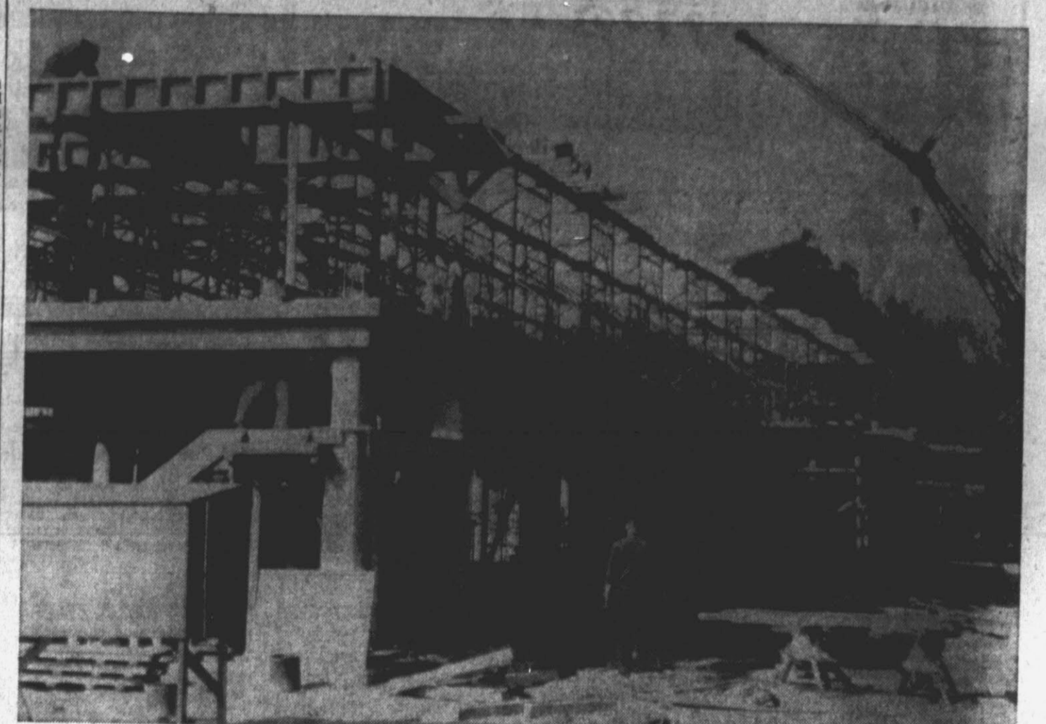
GOING UP—Workmen prepare to pour concrete for the second floor of the new men's dormitory which is now under construction on the new section of the ECC campus. Above is shown one of the "H" shape buildings. It will house more than 600 students and will have its own cafeteria facilities. (Reflector Staff Photo)
