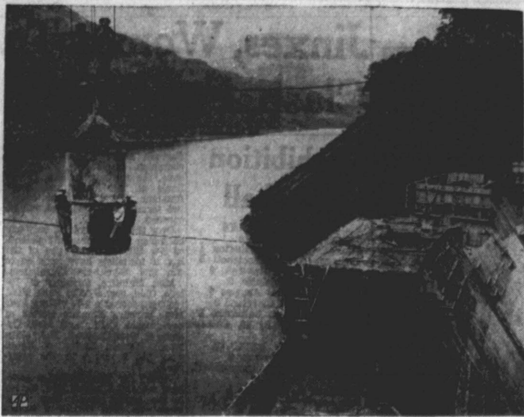
AERIAL APPROACH —Concrete bucket serves as lofty conveyance for workers moving along the giant Wu-Sheh Dam under construction in mountainous terrain of central Formosa.
