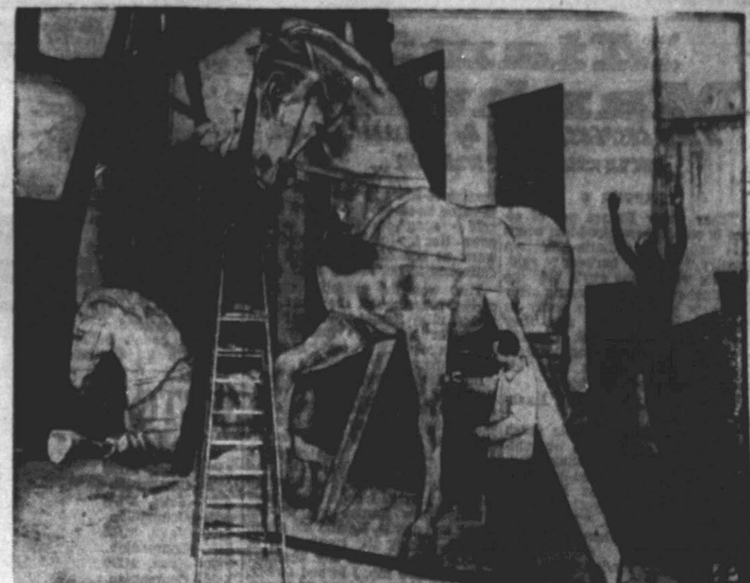
REMOUNTS FOR THE GATE — West Berlin craftsmen work on new copper harness to draw the new chariot which will rest on top of the Brandenburg Gate. The famed Berlin landmark is astride the dividing line between the eastern and western sectors of the city.
