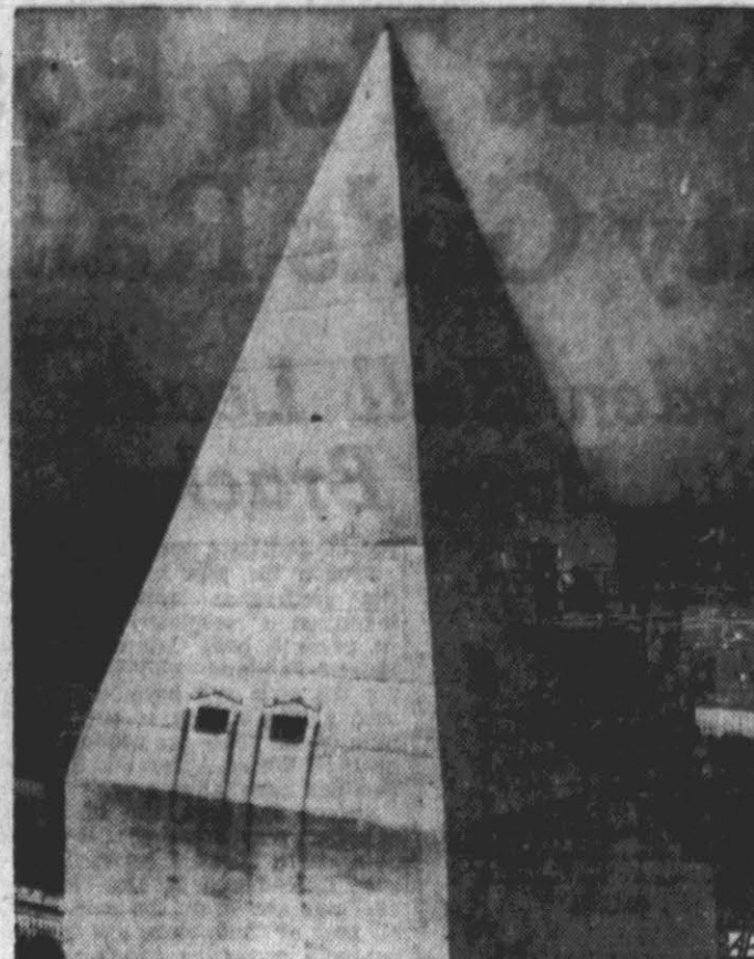
LOFTY WARNING —Workmen stand on temporary framework near peak of the Washington Monument to install a new lighting system which will warn off aircraft. View of peak, 555 feet 5/8 inches above the ground, was made from helicopter.
