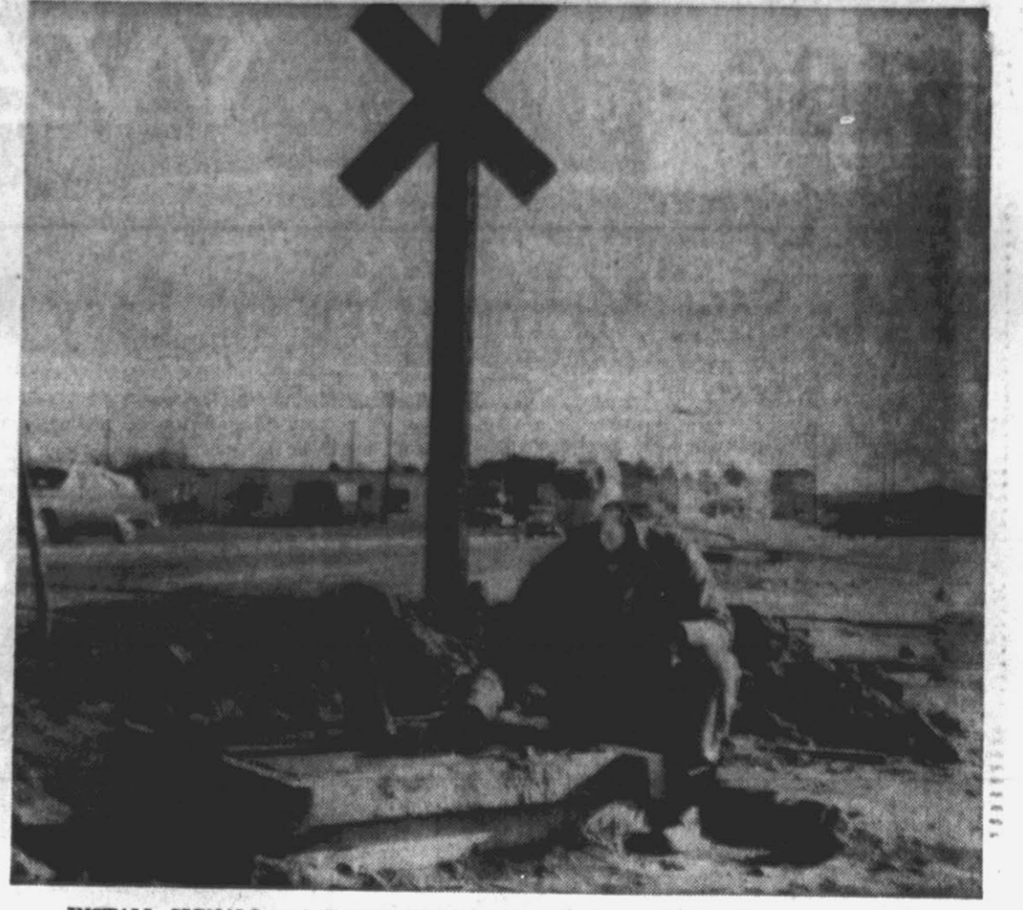
INSTALL SIGNALS —A Norfolk and Southern workman installs the concrete base for blinker lights at the railroad crossing on Memorial Drive. Warning lights are being installed in the islands of the four-lane drive and automatic gates are to be placed on each side of the road. The barriers will lower themselves to block the highway as a train approaches. (Reflector Staff Photo)
