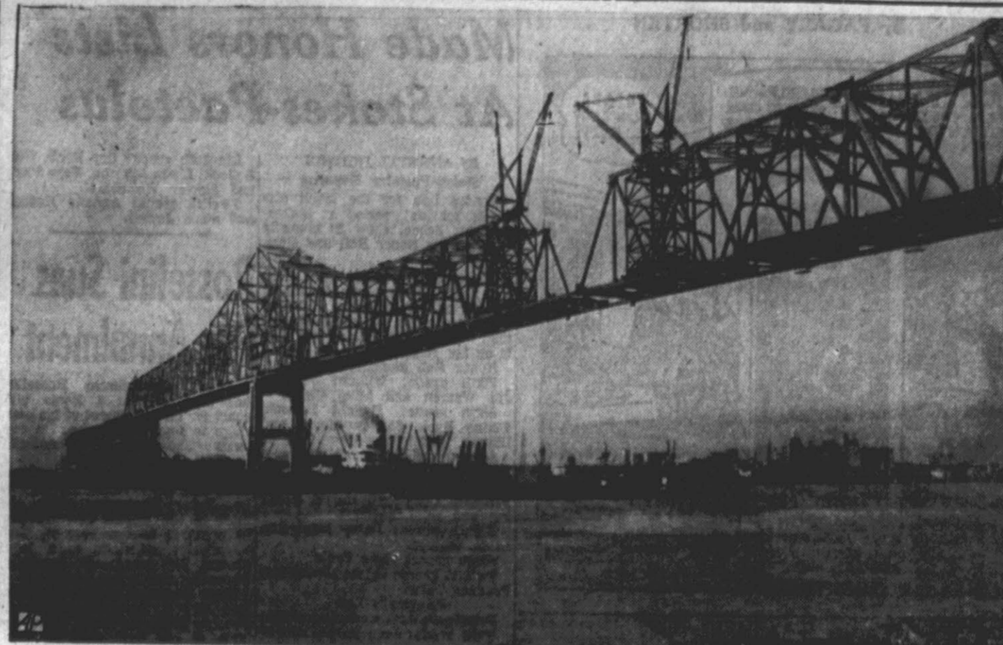
MAKING THE ENDS MEET — Derricks place 36-ton, 100-foot steel beams in place to join two sections of cantilever bridge over Mississippi River at New Orleans. Sections were constructed from each bank toward center of the river.
