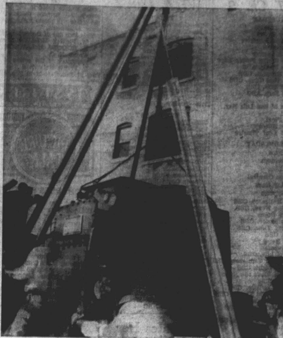
Problem was to place this transformer
