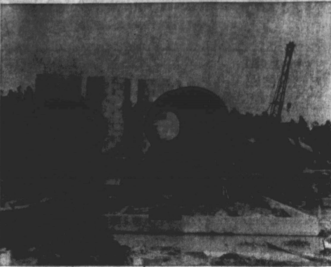
DRYERS BEING PLACED ON FOUNDATIONS . . . To Handle Wood Shavings From Silos In The Rear.
