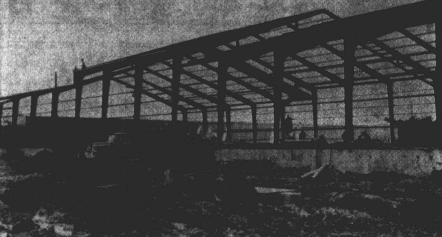
STEEL FRAMING COMPLETED ON MAIN PRODUCTION BUILDING . . . At Multi-Million Dollar Flakeboard Plant at Farmville.
