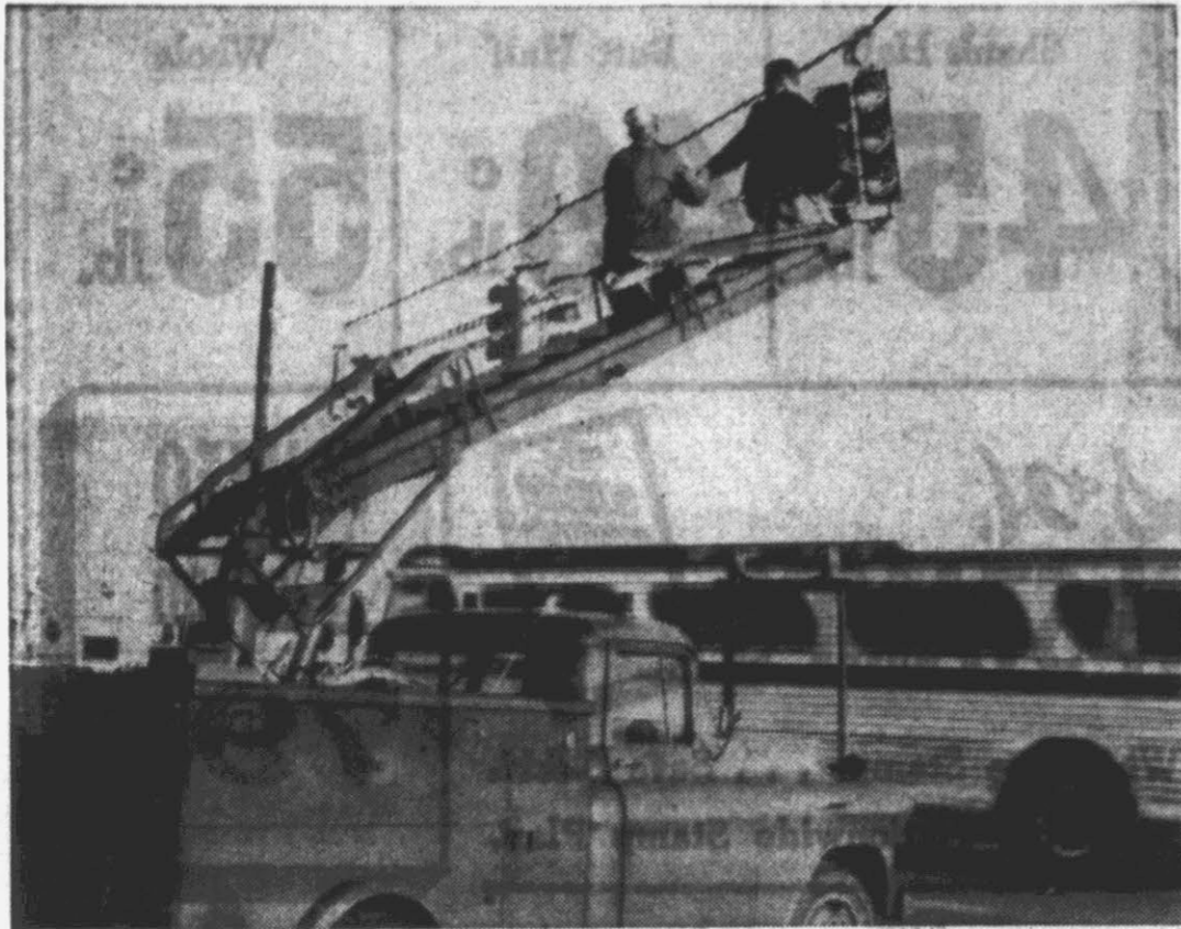
NEW TRAFFIC LIGHTS—State Highway Department technicians make final adjustments in traffic lights which have been installed at West End Circle to control traffic on the new bypass and U. S. 264 Traffic actuated lights are also being installed at the bypass intersection with N. C. 43 near Pitt Memorial Hospital.
