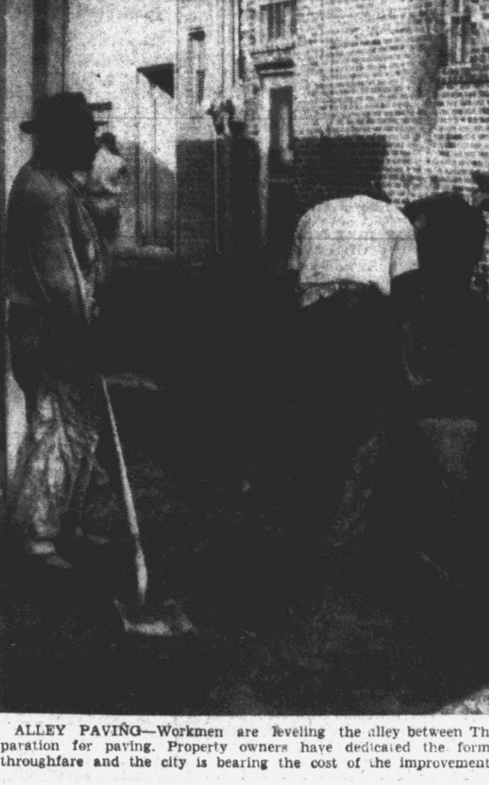
ALLEY PAVING—Workmen are leveling the alley between Third and Washington Sts. in preparation for paving. Property owners have dedicated the formerly private alley as a public thoroughfare and the city is bearing the cost of the improvement. (Reflector Photo).
