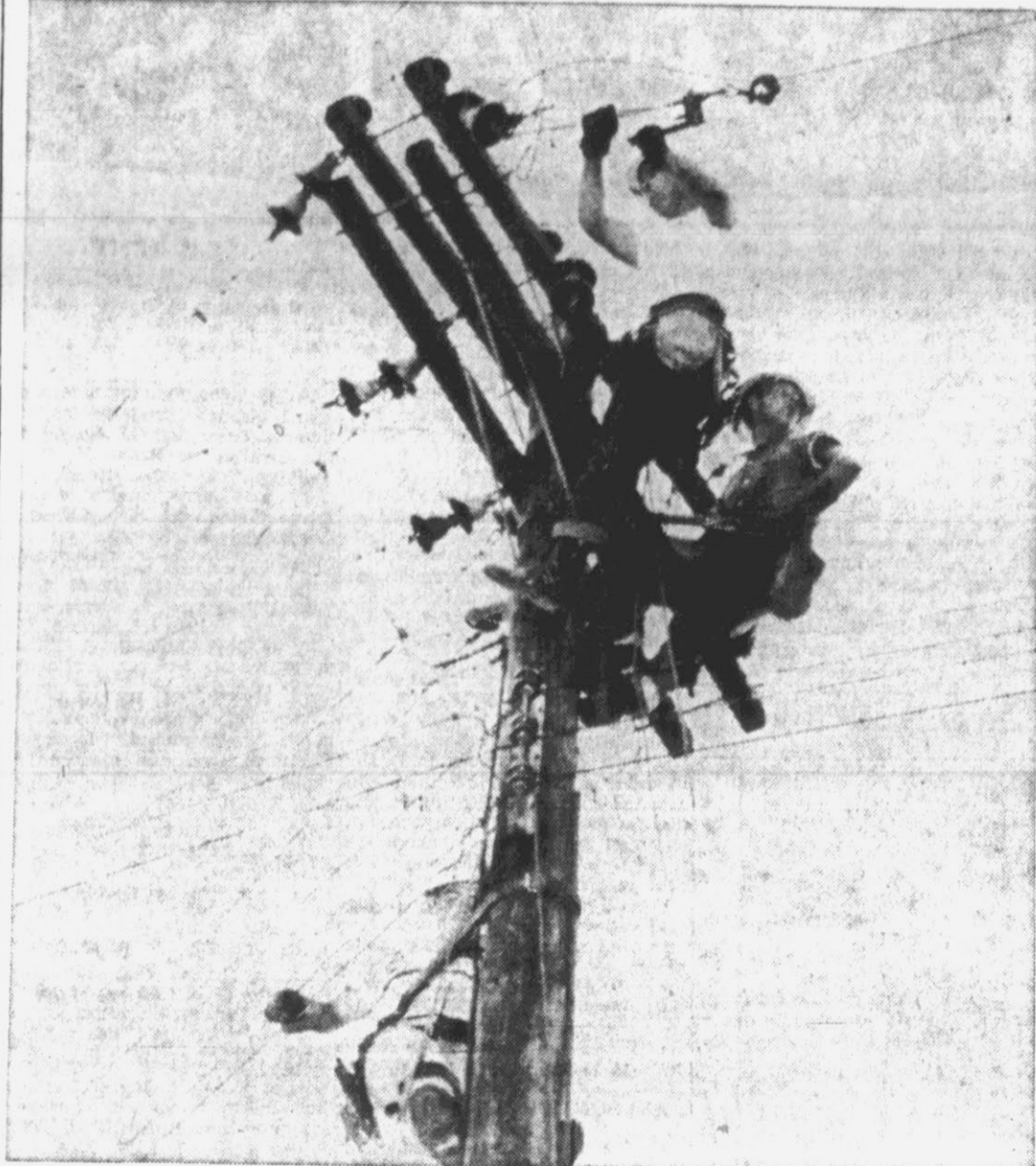
COLLISION BREAKS MAIN CIRCUIT ... crews splice lines to restore service.
