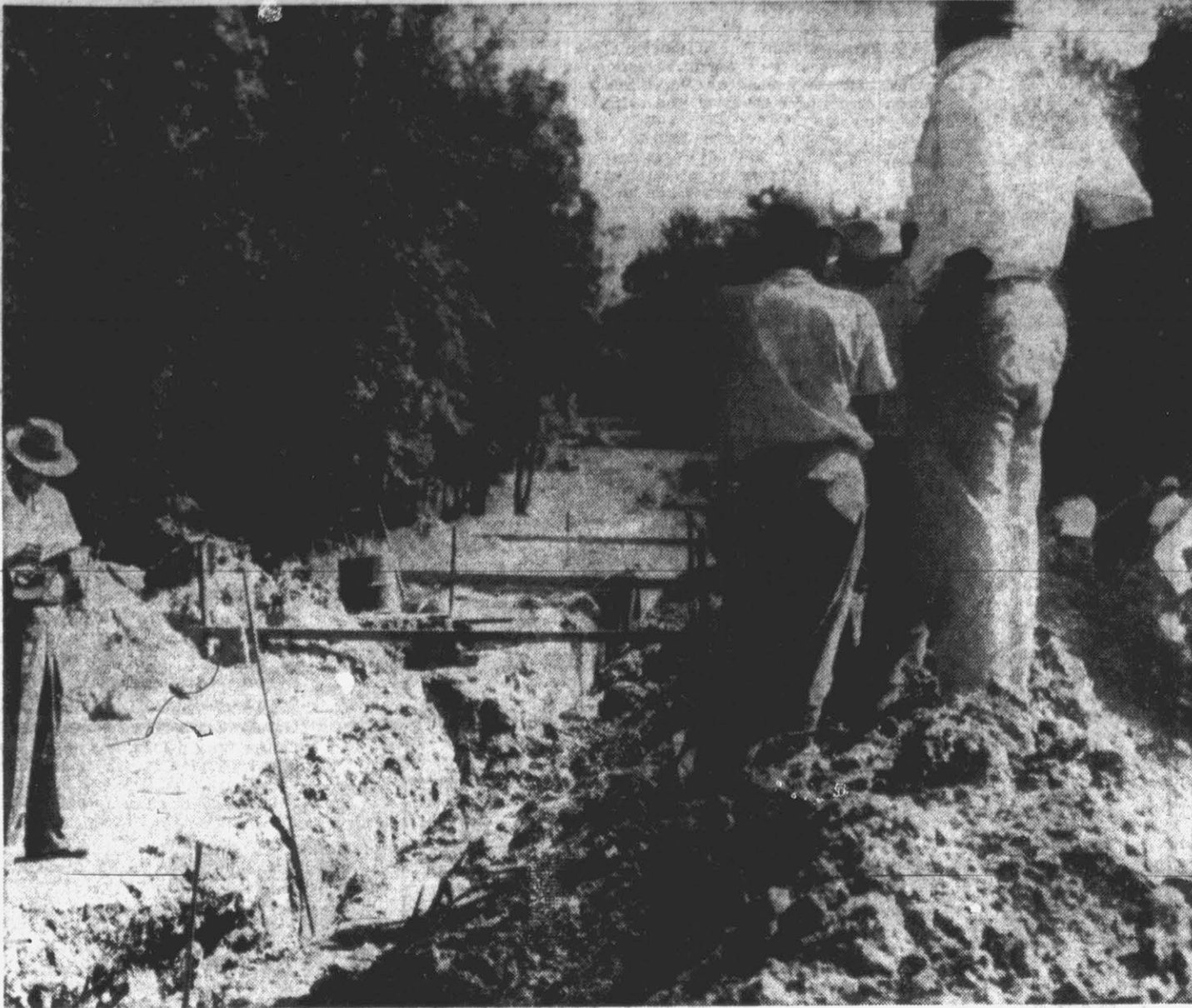
Wall of ditch collapsed on Utilities worker . . . Archie Williams died instantly.
