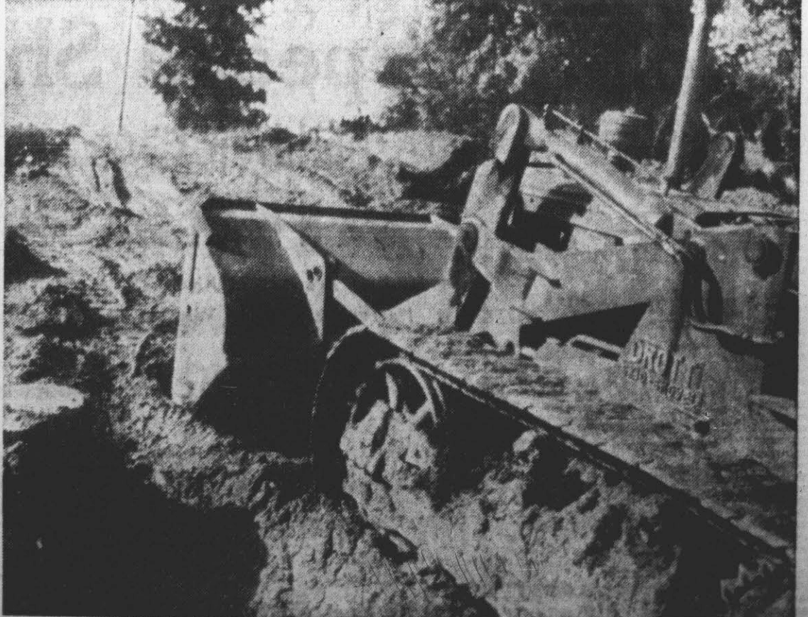
ELM ST. OPENING—City crews are extending Elm St. from its present deadend to the U. S. 264 bypass. Above a tractor-shovel is shown at work on the fill needed for the street extension.
