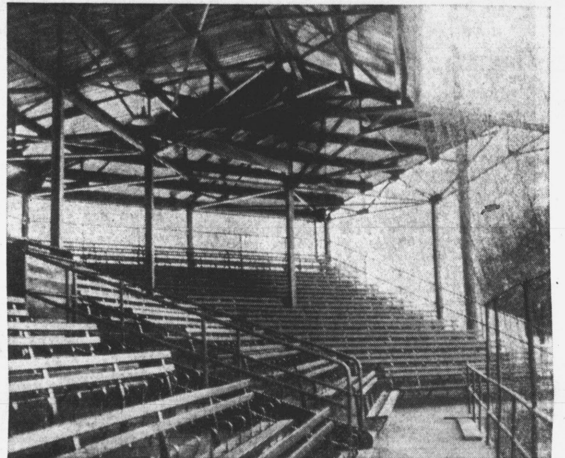
NEW LOOK —Over 250 gallons of paint have been used by workers who have been painting at the ballpark for several weeks. It took a considerable length of time to clean the bird nests from under and around the steel beams and seats. The wire backstop is in excellent condition.
