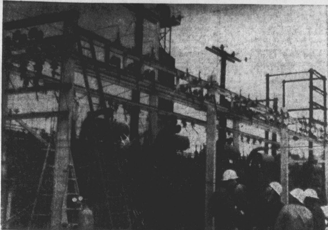
MAN BURNED—Utilities linemen look over the substation on which William B. Ebram, Negro Utilities employee was working yesterday when he came in contact with high voltage wires. Ebram was working on the ladder shown to the left above. The top of the wooden ladder was charred and insulators to the right of the ladder were broken. (Reflector Photo by Alvin Taylor).
