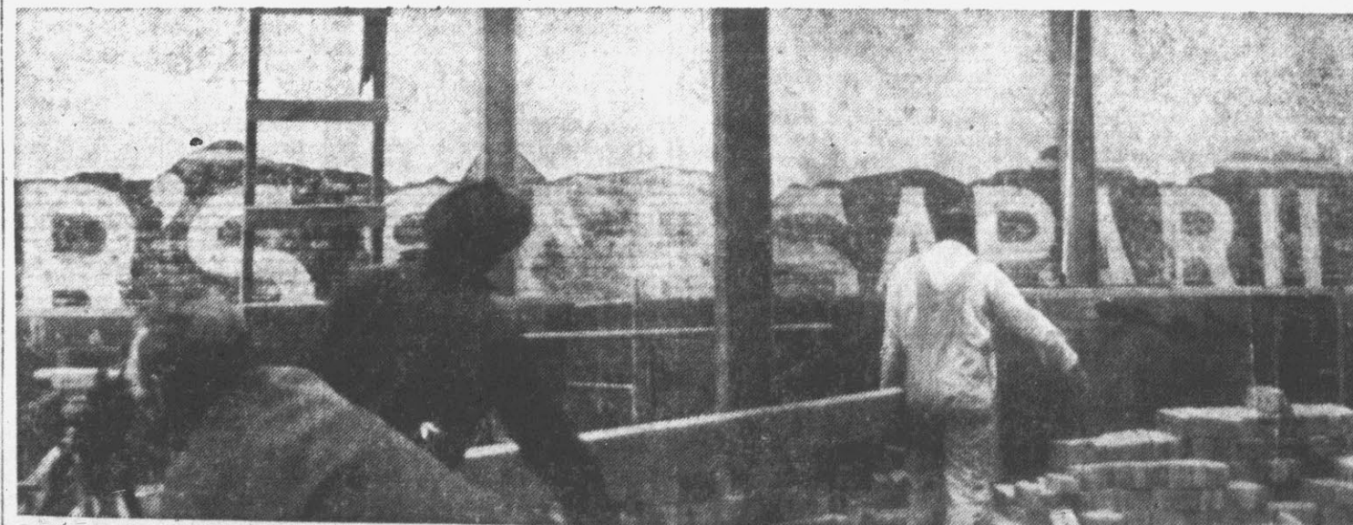
ANYONE FOR SARSAPARILLA—The above sign, believed to be over three-quarters of a century old, was uncovered by workers who are constructing a new building here on Evans Street.
