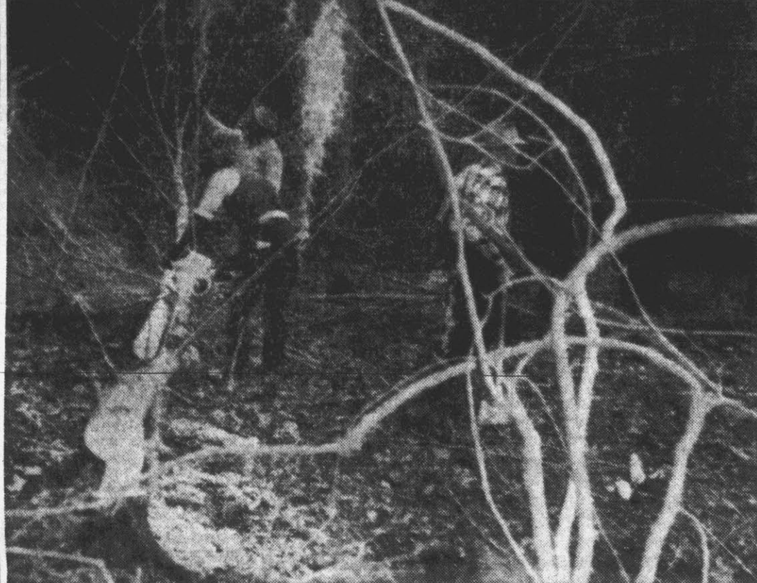
CUT TREES—Chain saws are whining in the low area along Greene Mill Run as workmen clear a right-of-way for the stream. The workers started at the mouth on the Tar River and will work back to N. C. Highway 43. The work is expected to eliminate flooding along the stream within the city. (Reflector Staff Photos).
