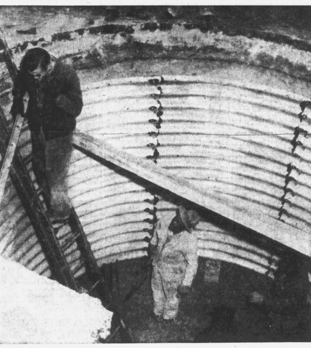
UNDERGROUND ELECTRICAL SYSTEM —Workmen are shown above as they work on a distribution manhole on Fifth St. between Five Points and Washington St. A new idea in construction is being used on the project. Galvanized steel walls are being used in the place of concrete or brick walls. (Reflector Staff Photo).
