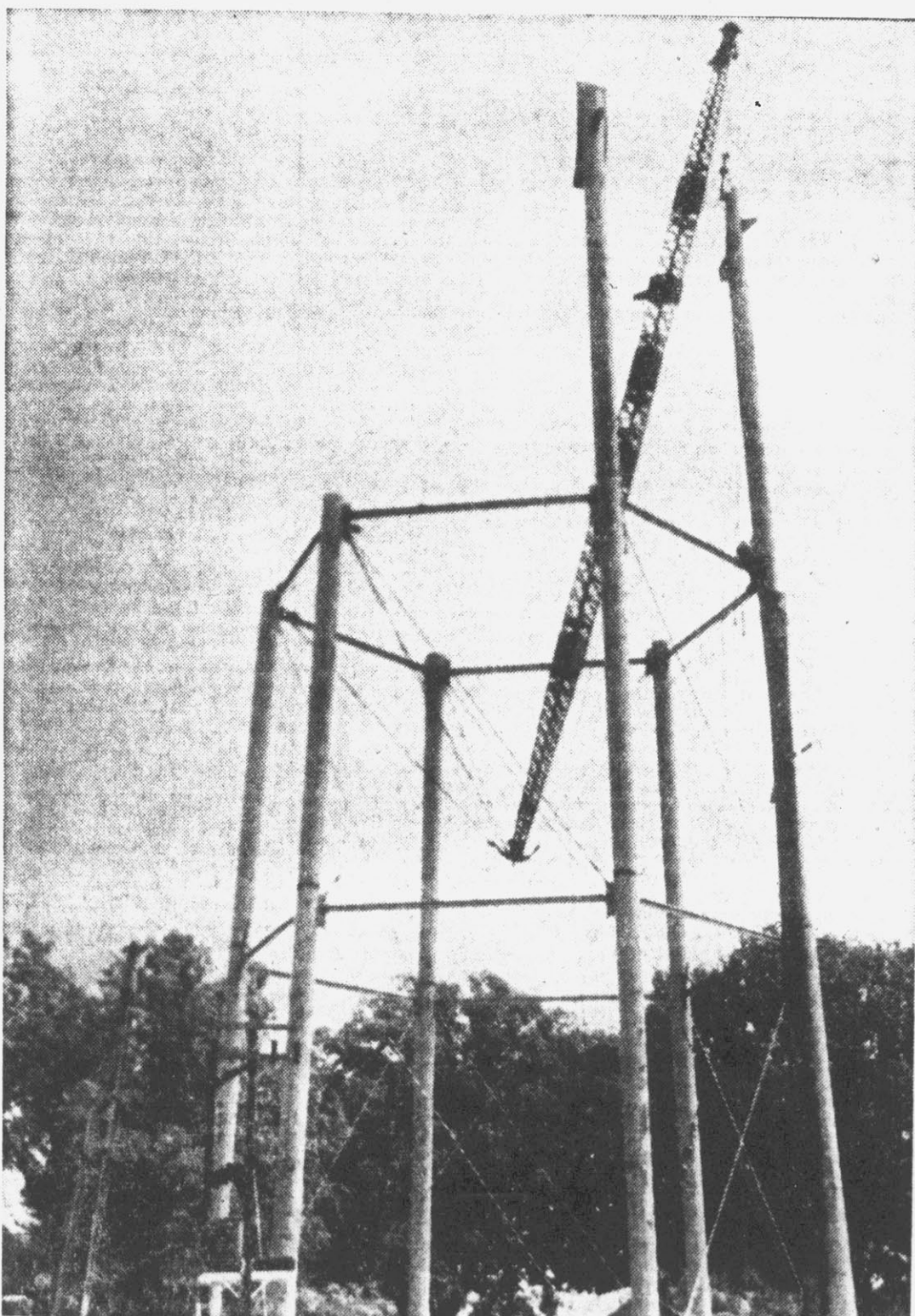
Ayden placed into operation this year a new 300,000 gallon capacity water tank. The new structure replaces an antiquated structure back of the Town Hall which will continue to be used for emergencies. Normal functions of Ayden's water department are being handled with the new tank which is a storage place for water drawn from two municipal wells.
