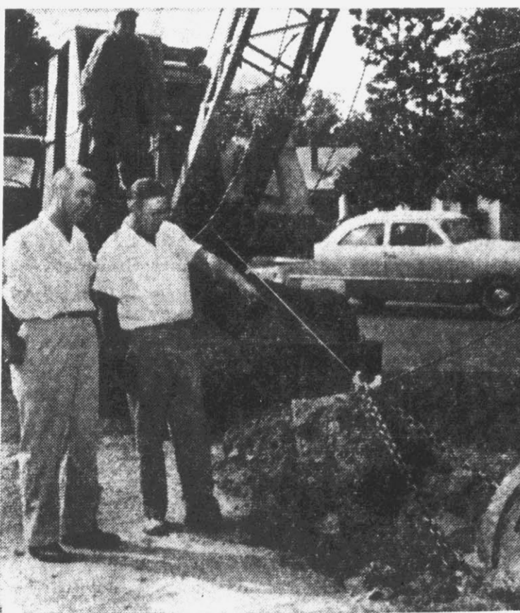
A $7,900 contract has been granted for paving and widening several streets in Ayden, including some private improvements under the inspection of the city. On the left Mayor Corey Stokes is shown checking with the paving foreman regarding some of the improvements. (Photo by James W. Everett).
