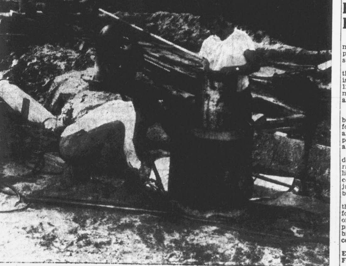
WATER WELL COMPLETED—Workmen above put final touches on the deep well which was recently completed at the Washington and 13th St. tank. The pump for the well which will deliver 1,200,000 gallons of water into the city's system is now on order. (Reflector Photo by Alvin Taylor.)
