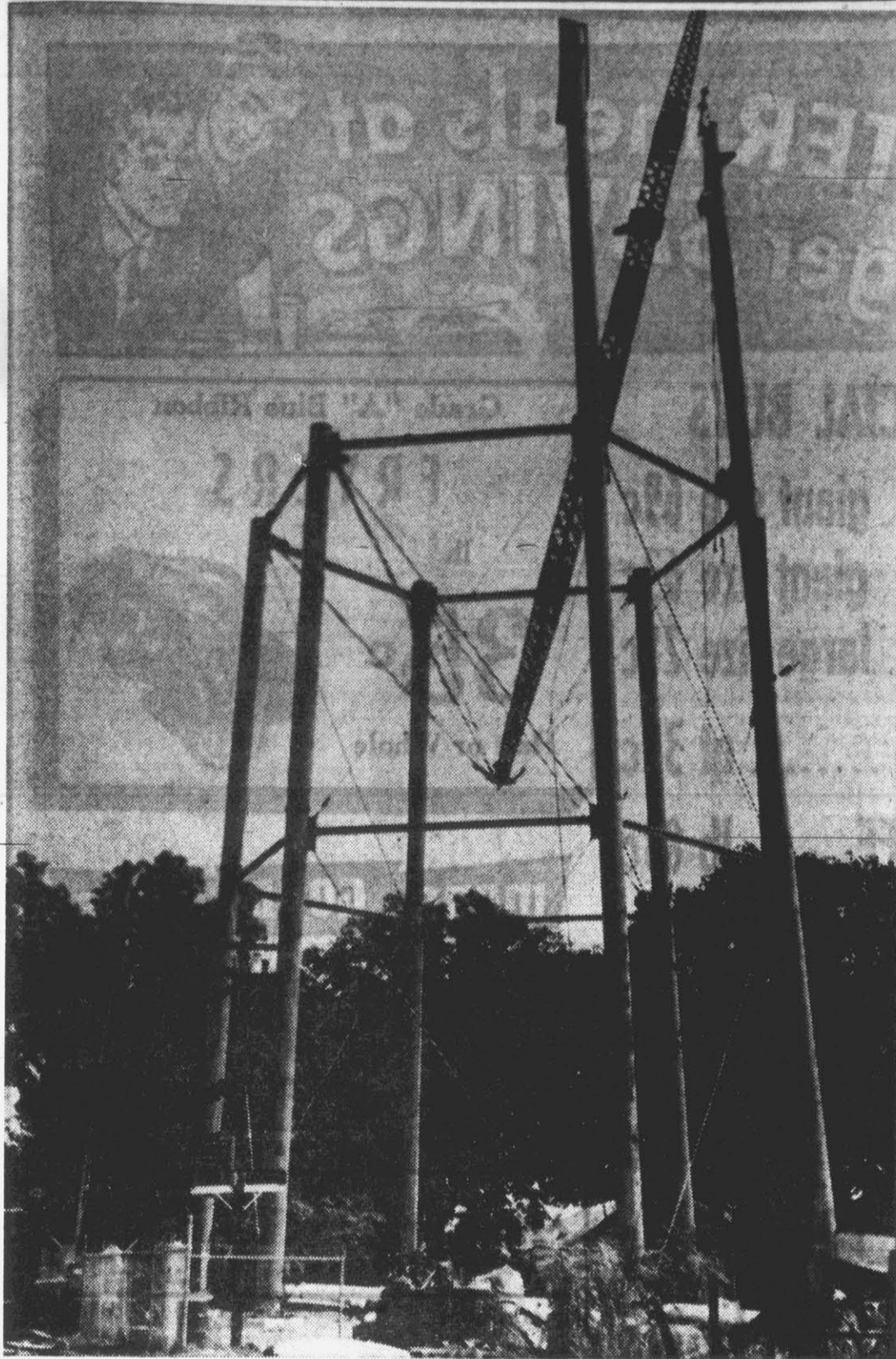
The 100 foot tower which will support Ayden's new 300,000 gallon water tank is rapidly nearing completion. Structural steel work on the tower was started last week and the tank is expected to be put in use in the early fall. (Reflector Staff Photo).
