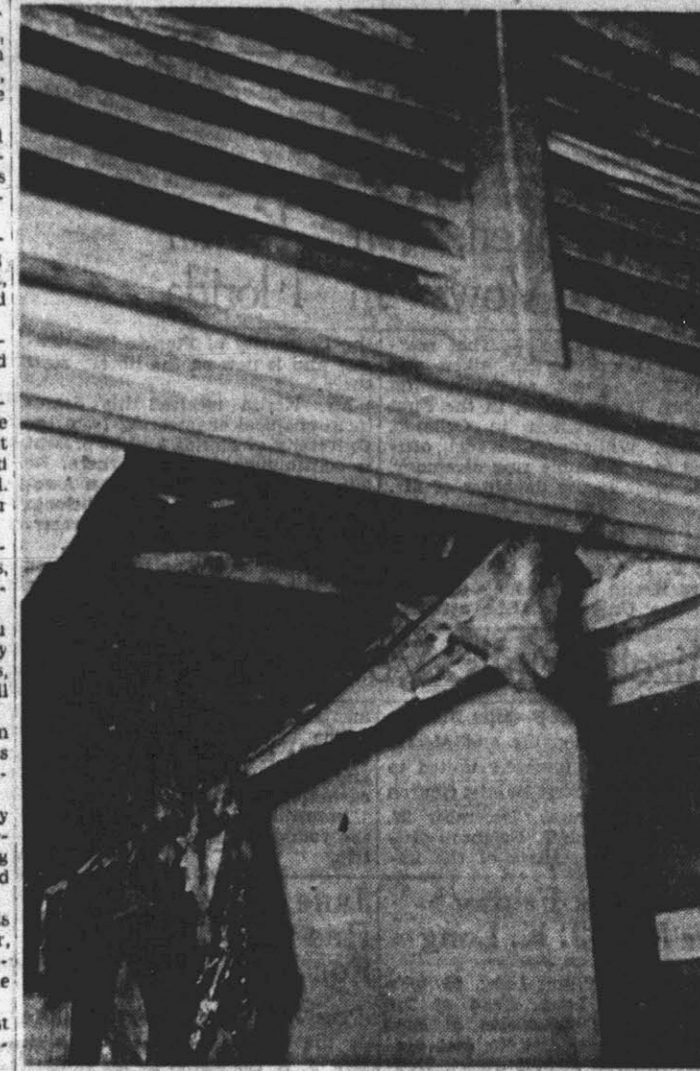
AFTER ROOF COLLAPSED — A jagged portion of the clinic roof dangles into a hallway after it gave way from flames that gutted the structure shortly after 5 a. m. today. Damage to medical equipment in the building was feared heavy though the brick exterior was left standing.
