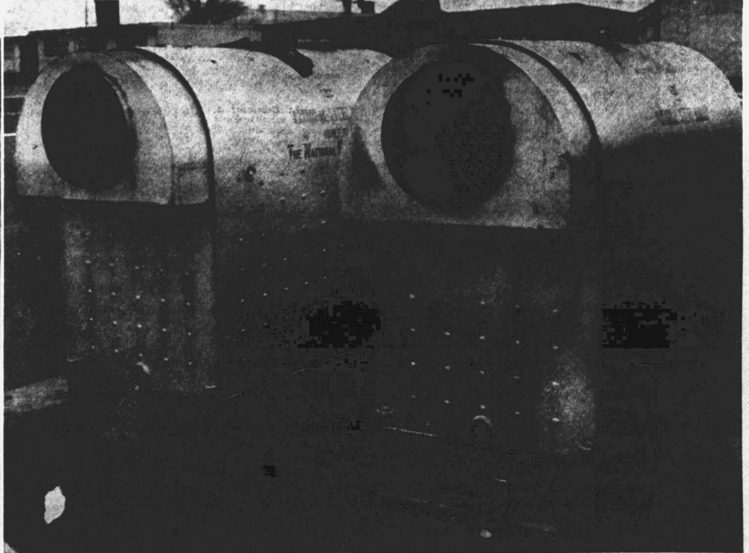
It will be warm in Greenville's new high school when the building, now under construction on Elm St., is completed. The two big boilers shown above were recently placed in position in what will be the boiler room of the school. Concrete floors and walls in that section of the building was poured some time ago. (Reflector Photo by Alvin Taylor).
