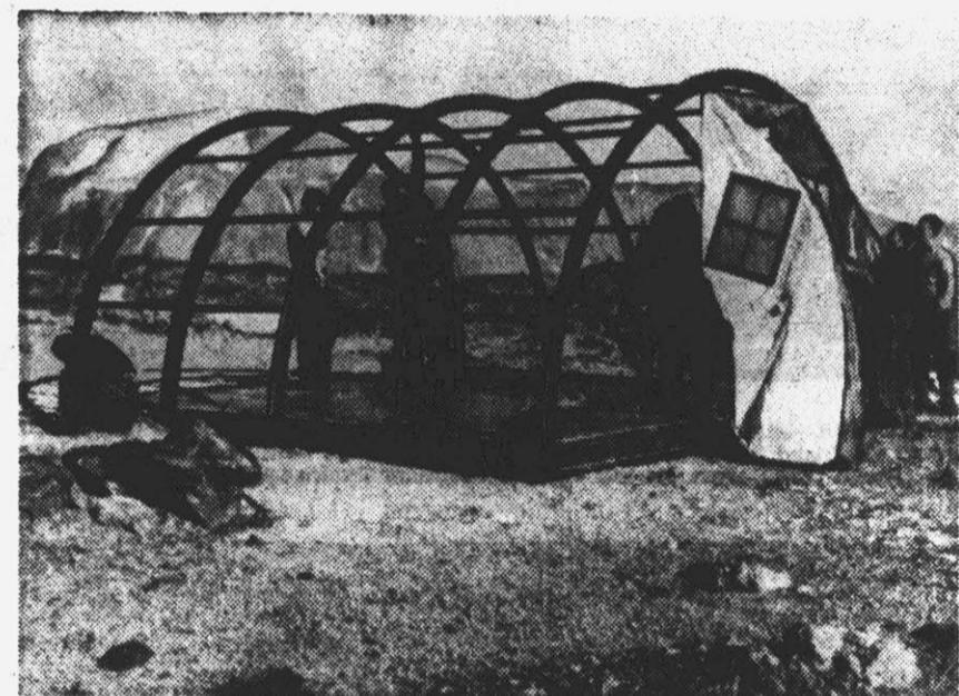
Crew members set up prefabricated hut at Arctic defense post. It will be used as living quarters for Air Force personnel.
