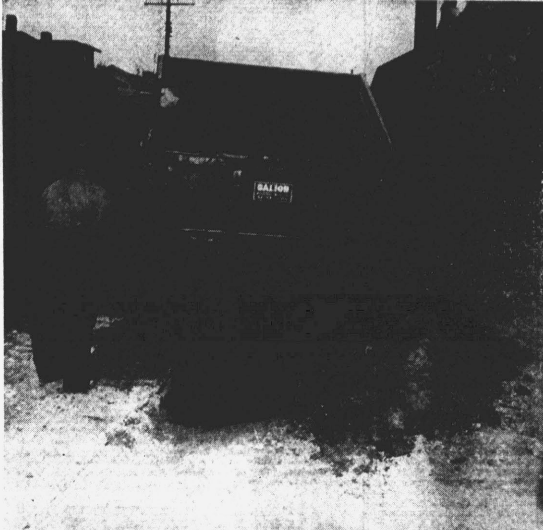
Workmen above pour a new soil base for paving on Pitt St. Additional work was required on the job because the newly installed paving for the street widening project was placed too low. City Manager James S. Hughes said the engineering firm which handled the job has agreed to bear the cost of the corrective work. (Reflector Staff Photo).
